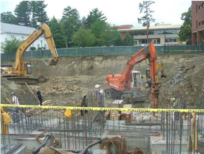
Figure 4. Photograph of the digging of the foundation for the South Academic Building. Possible materials that could be diverted from disposal in this photograph include concrete, wood beams, metal piping, copper wire, and plastic packaging. See Table 1 for a more comprehensive list of construction and demolition debris.
