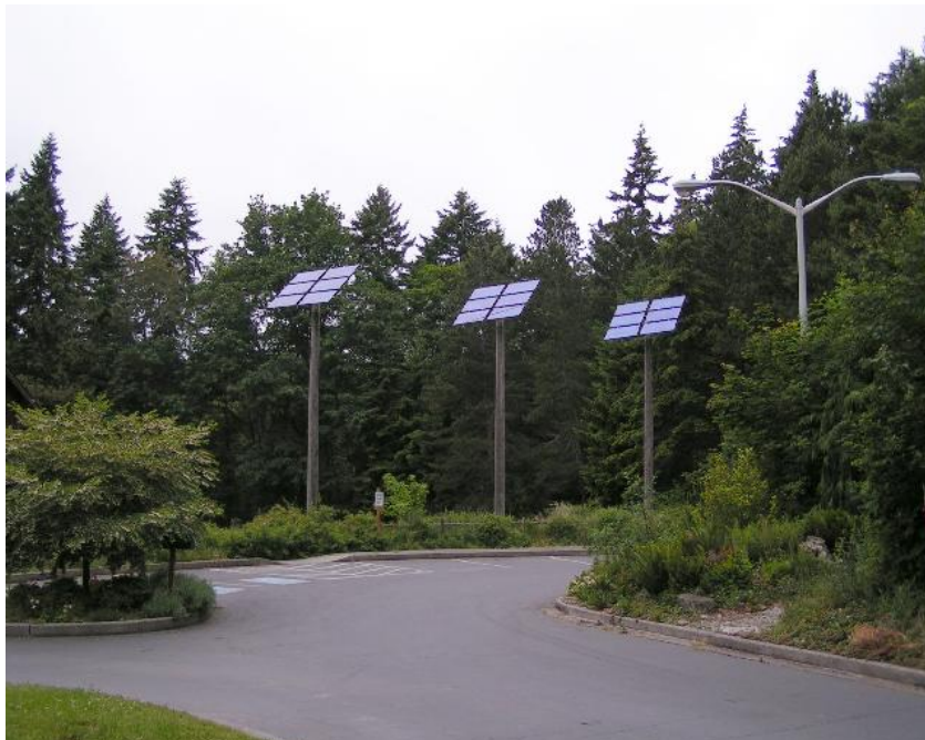
Figure 7. A representative PV pole array in a wooded area similar to the Dodd Circle.
